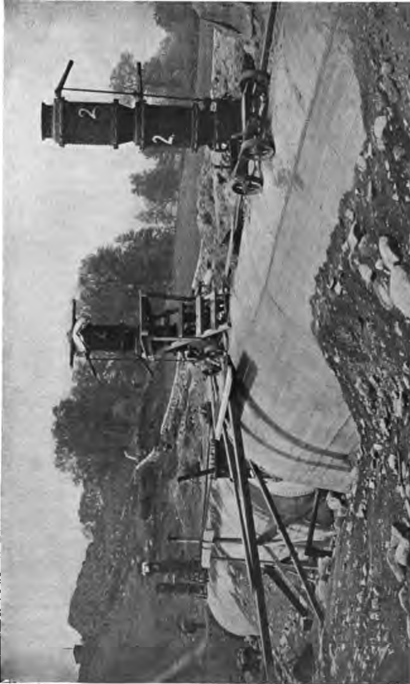
PLATE 160.—Contract 68. Hunters Brook Steel Pipe Siphon. Apparatus for mixing and placing mortar lining with "cement gun" mounted on outside lining of steel pipe. Sand and cement were placed in compartments of these machines and blown by compressed air through pipes to nozzle where water was added to form mortar coat sprayed on inside of pipe.
